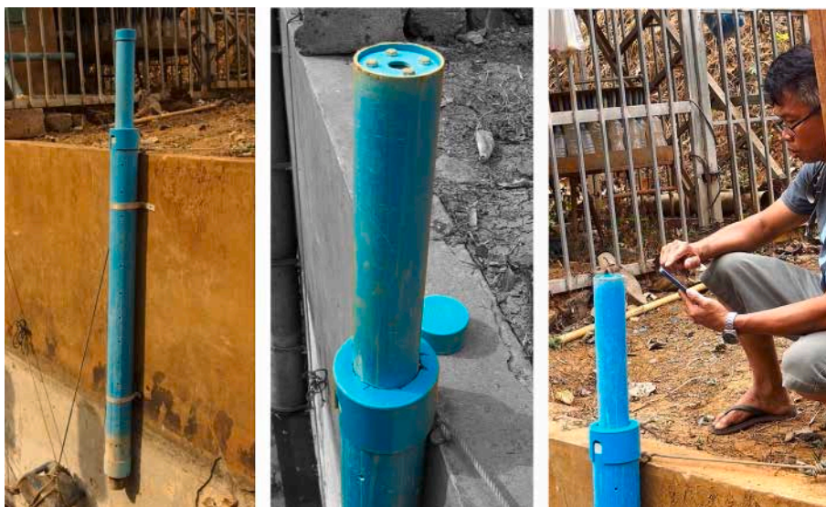
Fig. 19. Field deployment of the water level gauge for water level monitoring in a weir; a. Overall view of the complete device installed on the wall of a weir using wall mounting brackets; b. Top view of the gauge unit inserted at the upper end of the float guide tube #22 which is itself inserted into the strainer tube #25, the removable end cap (#21) for #22 is taken out and placed on the edge of the wall allowing access to the push-button cover assembly; c. Data downloading in the field using the Bluetooth Low Energy connectivity with Android app 'Serial Bluetooth Terminal'.
