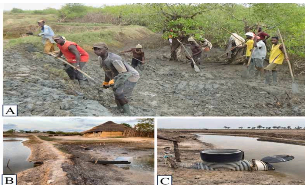
Fig. 7. Reinforcement of a collapsed main dike at Cafine (A); Palm trunk installed on a dike for water drainage at Elia (B); Water management tube installed on the main dike at Jobel (C).
