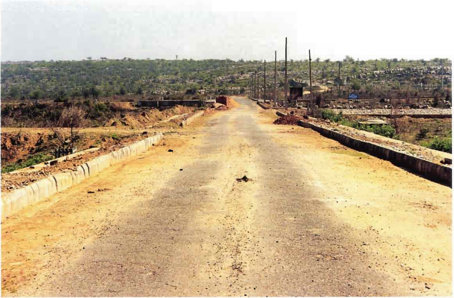
2 Tracts of land developed and ready to be built, near Gurgaon. Road traced in an arid landscape. Photograph: Ruchir Joshi 1999.
