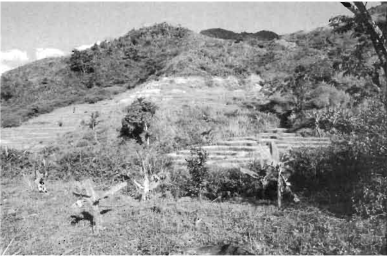
Fig. 18.3 Ambodivanana landscape: view of a Betsileo immigrant collapsed rice field terrace on foringa medium steep slope (source IRD-G. Serpantié) (see as color plate following Index )
